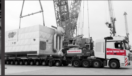
NAVOI NITROGEN BOILER (UZBEKISTAN)
